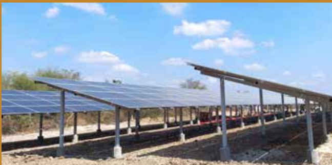
Partial view of the Photovoltaic Solar Park. UNISTMO. Ixtepec Campus
