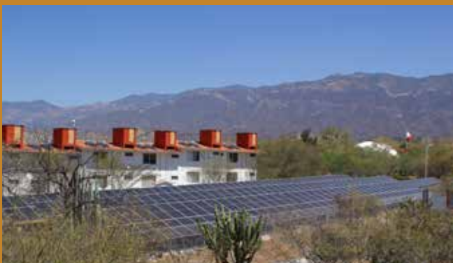
Partial view of the Photovoltaic Solar Park. UNCA. Teotitlán de Flores Magón
