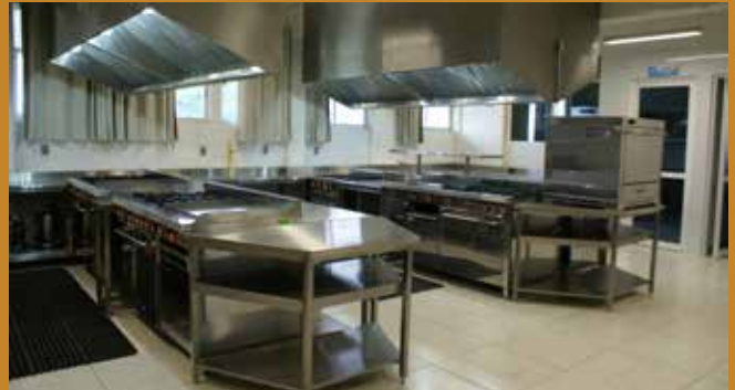
Partial interior view of the kitchen equipment at CINA. UNCA. Teotitlán de Flores Magón
